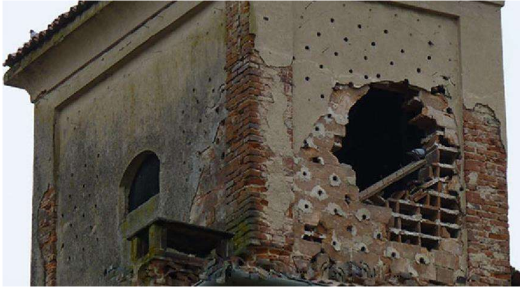
Figure 13: A ruined Sparrows tower. The collapse makes it possible to understand how artificial nests were made, buffering an empty space between load bearing structures
